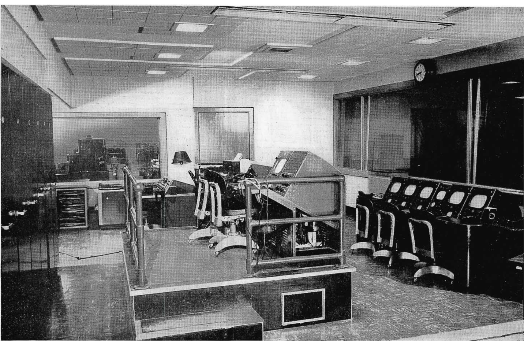
FIG. 13 (above). WBAP's television master control is combined with TV Studio #1 control as shown above. Five camera monitors (3 live, 2 film) and a preview monitor are on the lower level, next to the studio window. The program director and technical director sit on the raised platform. The TD, who does the camera switching, has a master monitor as well as the switching controls on his console. The audio operator sits at a floor-level console to the left of the program director (just behind the raised platform in this view).
